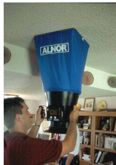
Figure 3. Testing for supply airflow balancing
